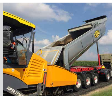
Tar surface finishing: With the tarpaulin closed, the asphalt retains its required temperature.
